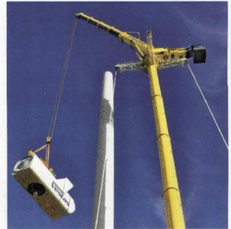
The GTK 1100 crane hoists the nacelle and hub to the top of the V90 wind turbine tower.
