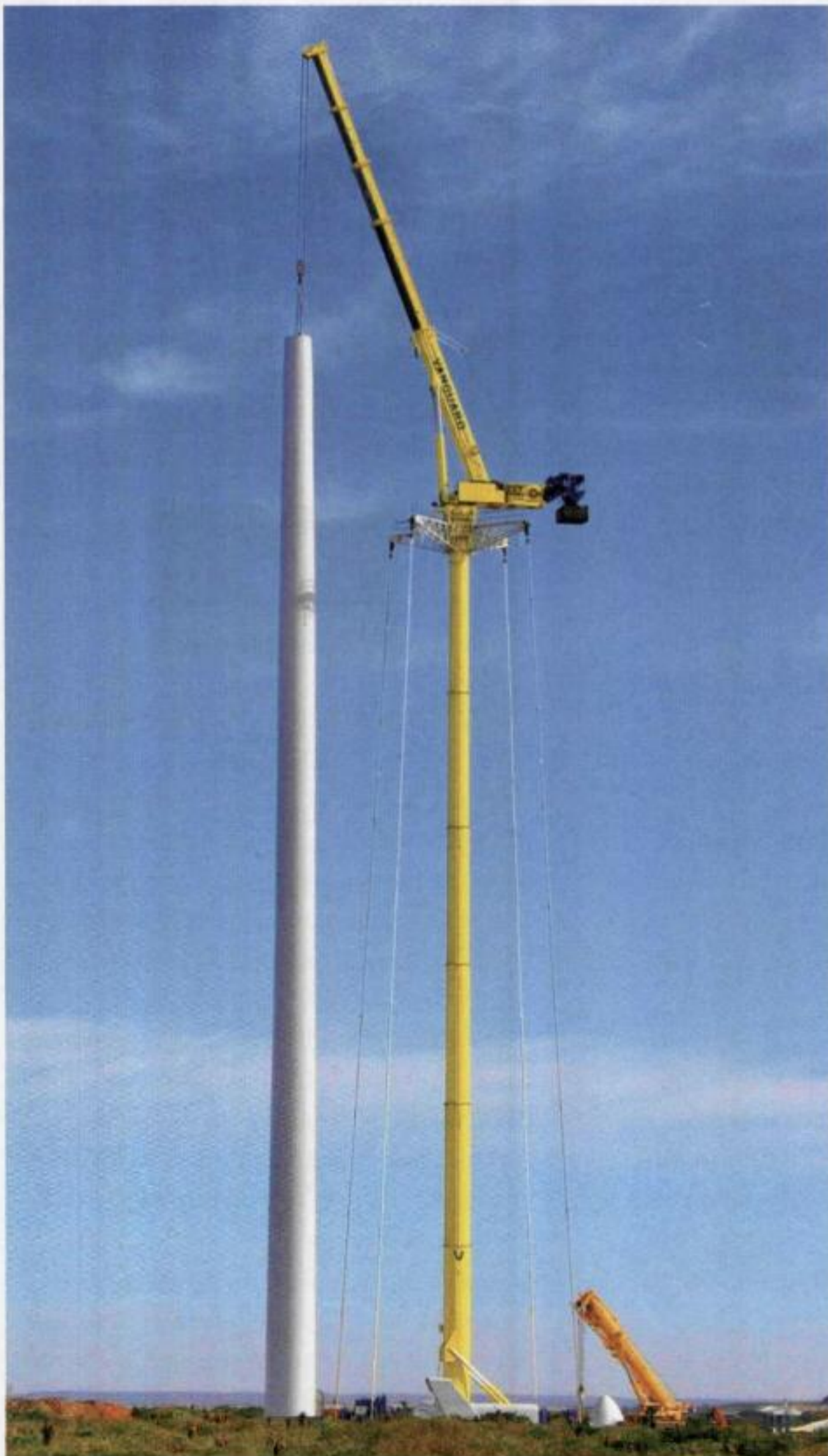
The tower sections of the V90 wind turbine are lifted into position by Vanguard's sophisticated GTK 1100 crane at the Coega wind farm.
