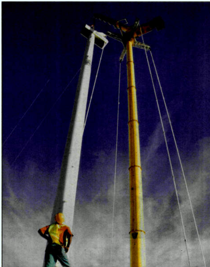
TO POWER PE'S WORLD CUP STADIUM. A worker looks on as the nacelle (a cover housing that holds equipment on a wind turbine) is lifted to the top of the first windmill at the planned wind farm in the Coega Industrial Development Zone with the help of the R70-million GTK1100 specialist windmill erection crane. The crane, a joint venture between Vanguard and Grindrod, can lift weights of 100 tons to heights of more than 100m. This first windmill is intended to power Port Elizabeth's Nelson Mandela Bay Stadium during the World Cup next month. Picture: Sabrina Dean.
